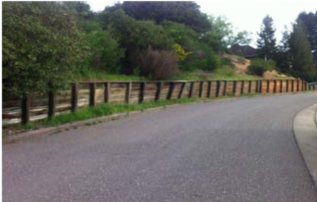
View to north, note failed section at center and apparently new section at far north.
