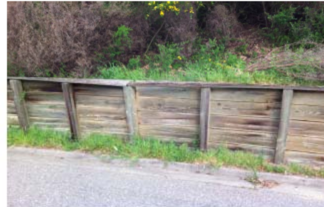
Close-up of failed center section, note lack of freeboard or drainage provisions.
