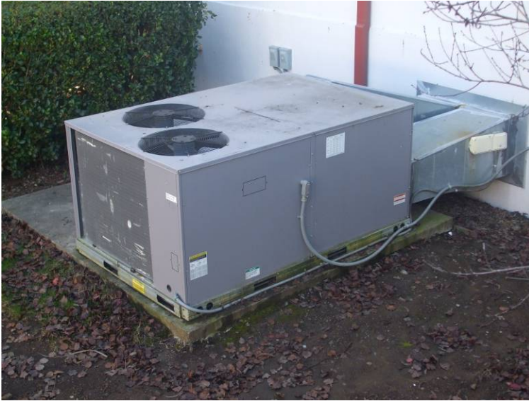
View of package air conditioning unit.
