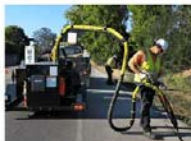
Janelle Wetzstein/Argus-Courier Staff This is a machine the city is renting to seal cracks in roads to keep them from deteriorating.
