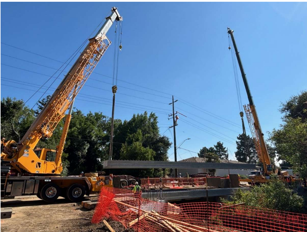
Figure 6 – Precast Voided Deck Slab Unit being erected into place by Bragg Crane.
