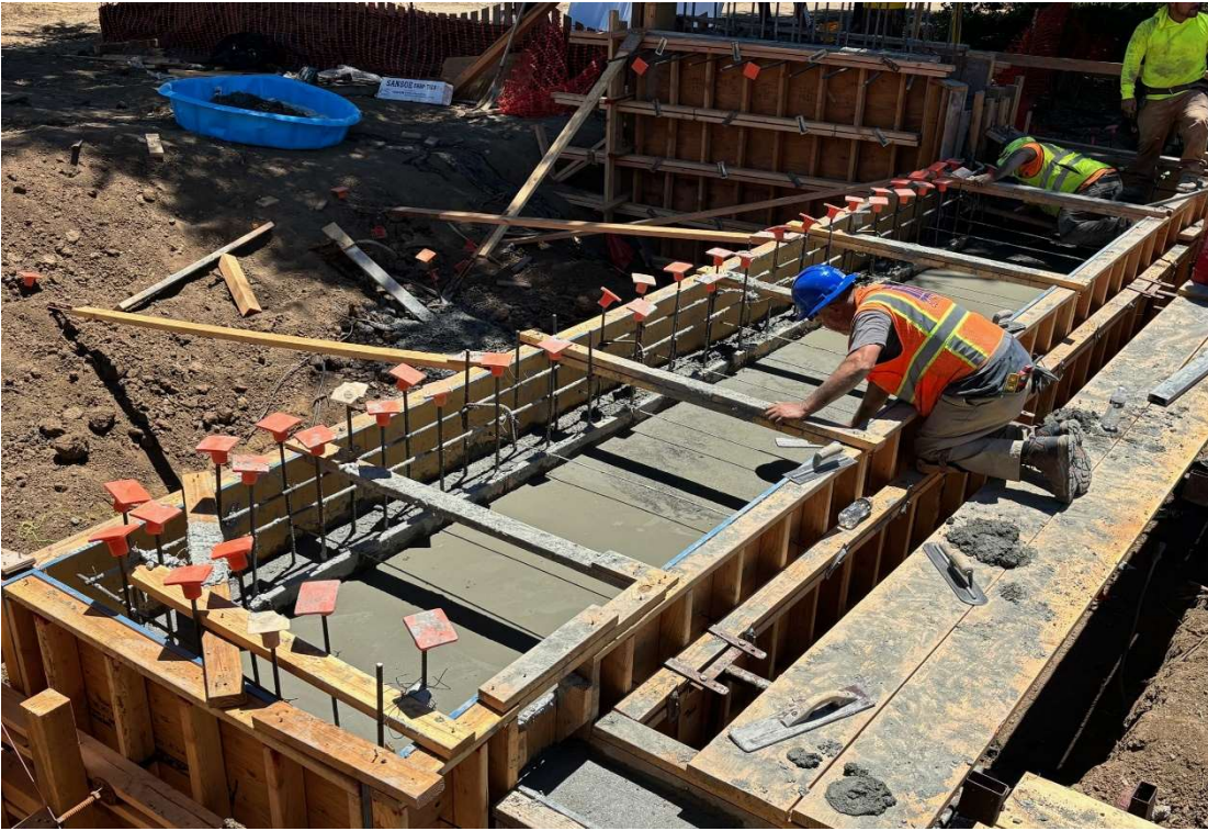
Figure 17 – Abutment 1 – Concrete Poured Out.
