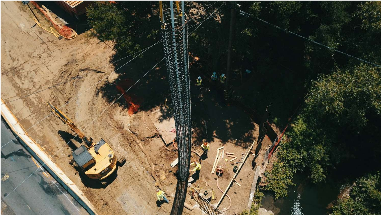
Figure 21 – Lowering the 49 ft cage in the drilled hole 3ft away from the Guy Wire.
