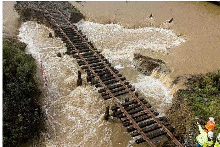
Figure 43: 2014 Levee Failure in Novato Source: San Francisco Gate
