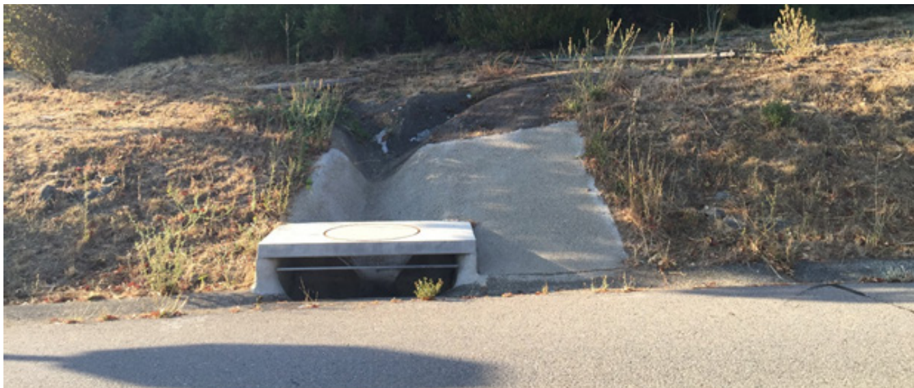
MVMCC has extensive v-ditch networks that will be mapped as part of this contract.
