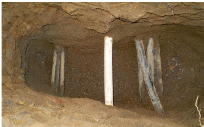
Previous potholing by Nute Engineering to determine the locations and depths of existing utilities on the MVMCC site.
