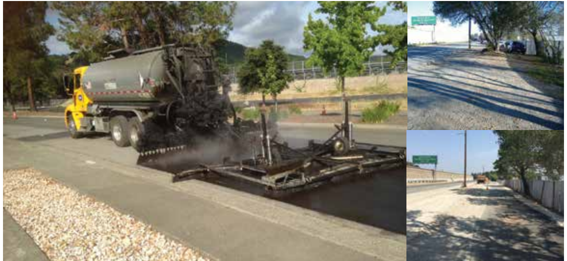
(Clockwise from left) 1. Resurfacing. 2. Nave Drive multi-use pathway, before. 3. Nave Drive multi-use pathway, in progress.
